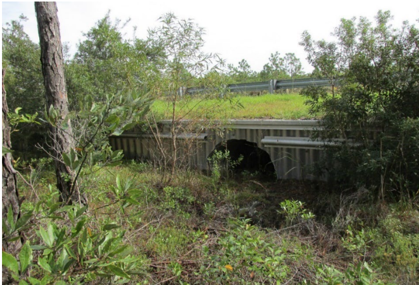
Figure 17. Culvert designed for small and medium animal passage on EF Middleton Blvd. Brunswick County.
